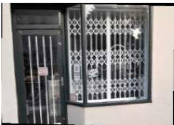
Security grilles installed internally.
